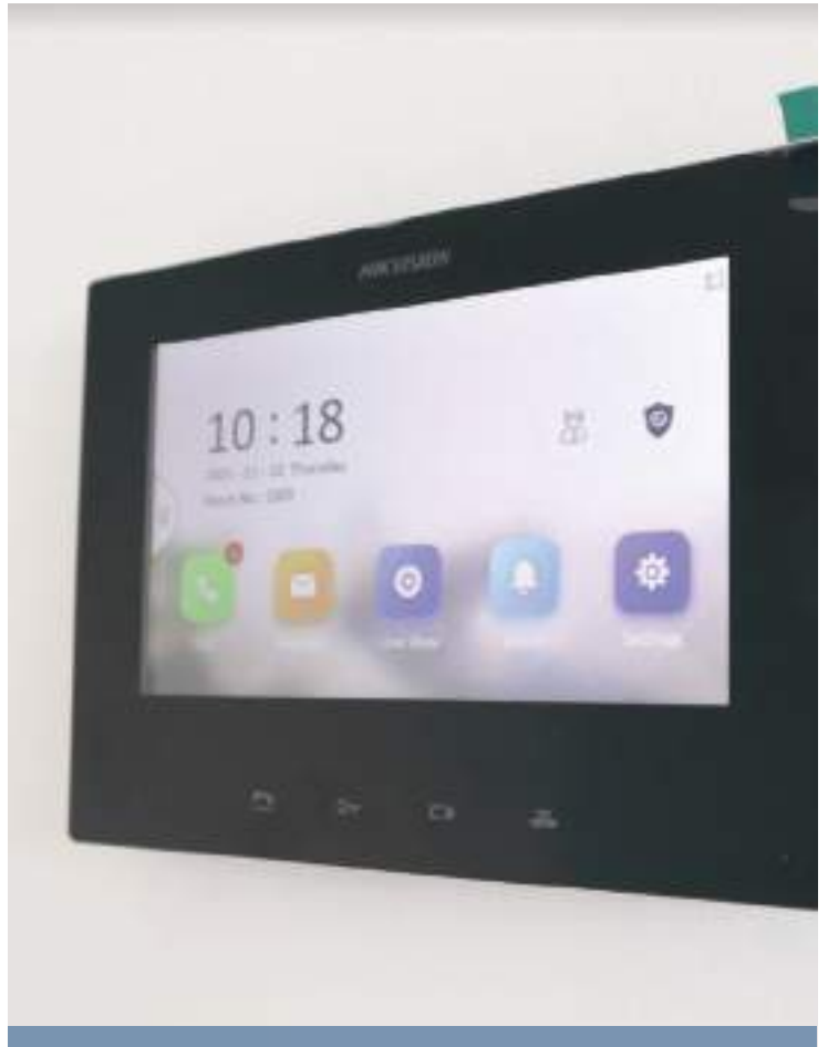
Intercom have been installed in each unit
